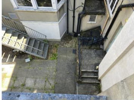
Fig. 4.48: The courtyard linking the Manor House, its rear extension and the 19th century barn.
